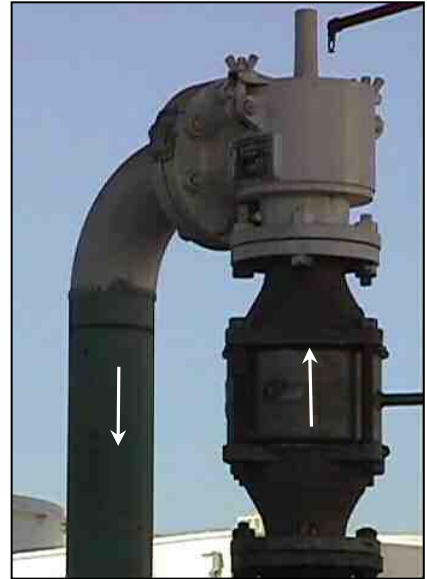
Hazard No. 8. Typical protected side restriction.
