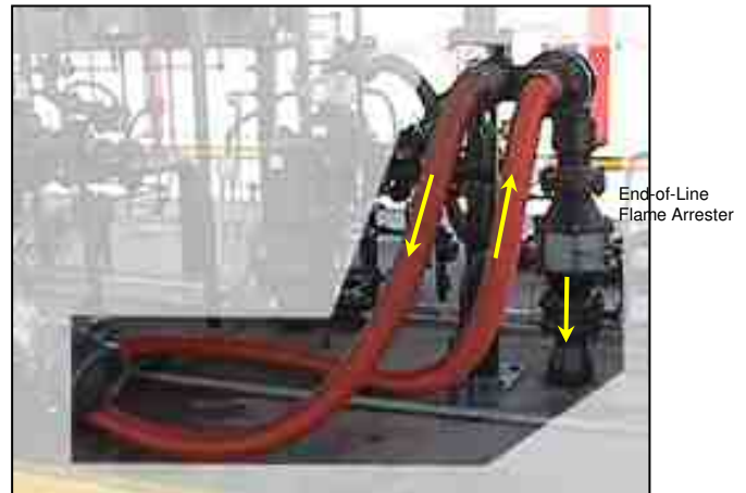
Hazard No. 2. Typical misapplication
