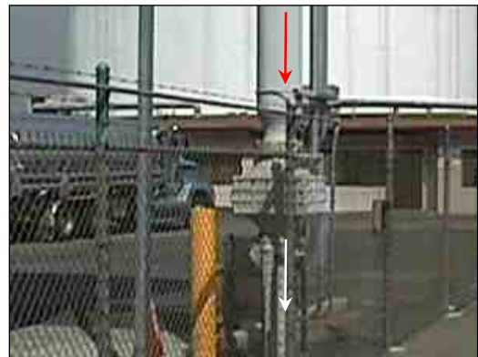
Hazard No. 7. Typical larger line size.
