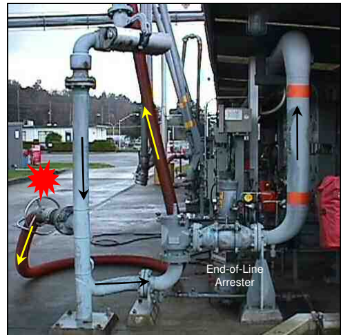
Hazard No. 6. Typical elbow and fitting.
